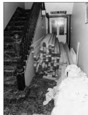
Figure 9: A blocked corridor with incorrect signage
